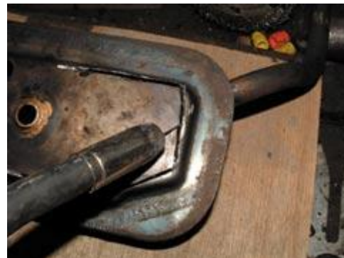
The tab has now been bent back into its original position and can be welded shut
